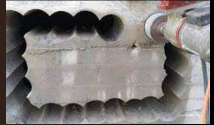
A.C. DUCT OPENING
